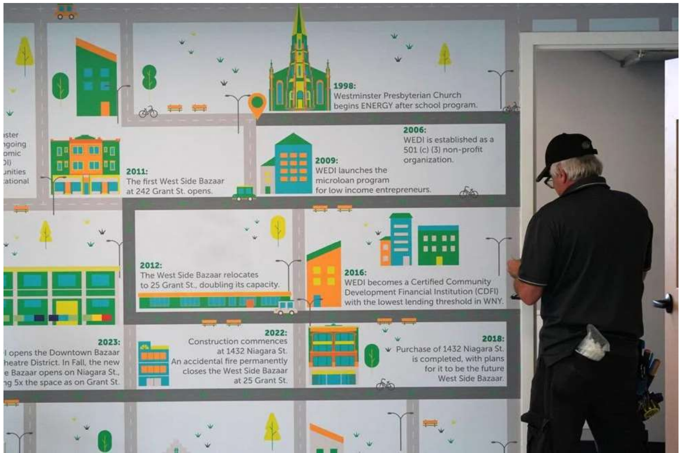
Mike Romeo of Amherst Alarm installs the access control for an office next to a mural in the new West Side Bazaar.
